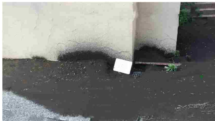
Figure 2-9: Sand boils on side of house in Kumamoto, showing volcanic material that was plastic and pumiceous in origin (Kayen 2017)
